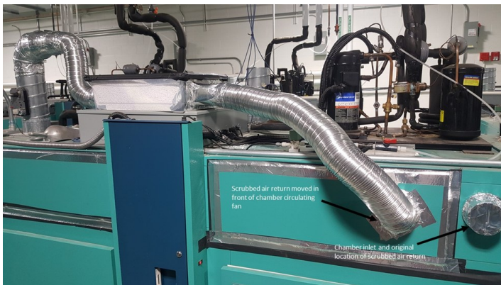
Figure 3: The location of the scrubbed air return was moved in front of one of the chamber's circulating fans in order to increase the flow of air through the soda lime box.
