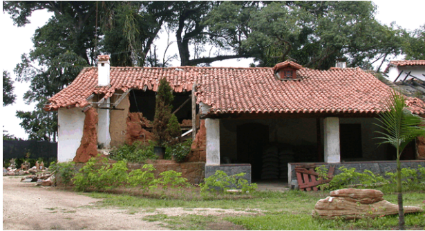
Figure 11. Main part of Casa Grande Velha – door behind porch opened to main living room. Roof damage on left side of image was from a tree that recently fell on CHTT's office (Suzana Rockhold, pers. comm.). Roof damage at far right was caused by fire.
