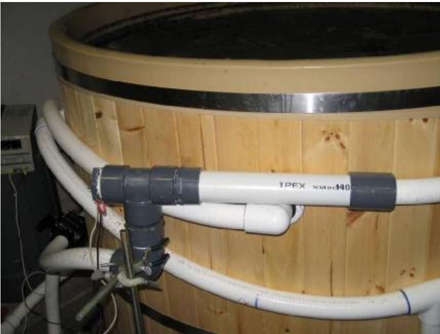
Figure 2. Electrodes mounted in configuration B (electrodes contained in an external bypass). The electrode unit is contained inside the horizontal pipe between the two grey fittings.
