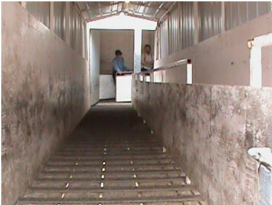
Figure 1. Covered hydraulic loading ramp with manway (looking down ramp from truck entry).
