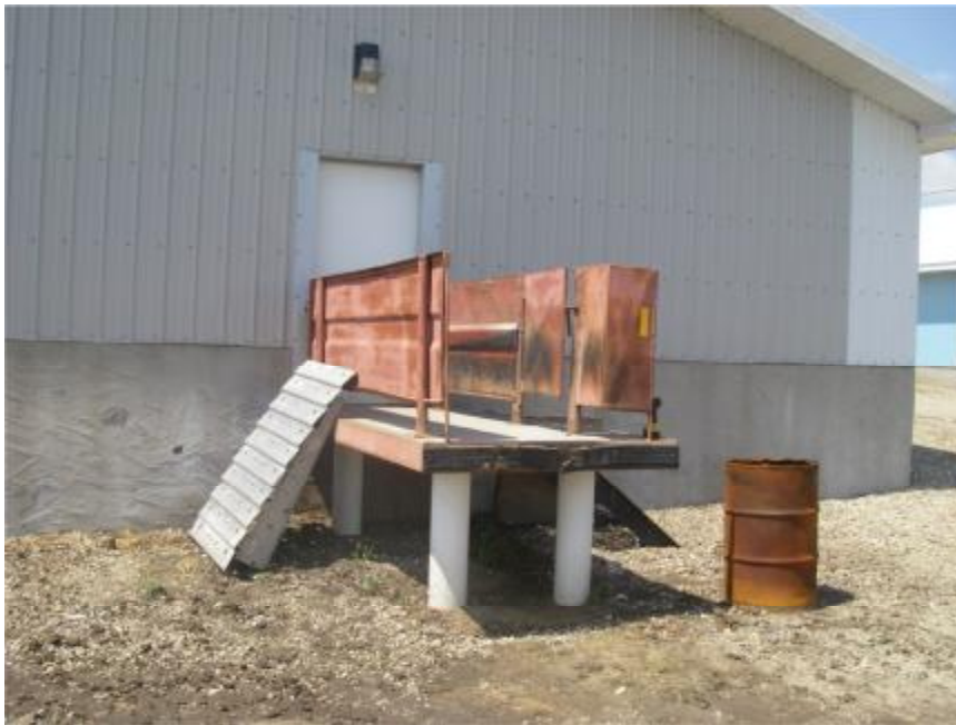
Figure 3. External loading ramp allows trucker to assist without entering barn. Note also the ramp extension (on the left) used to reduce the angle of internal truck ramp to the top deck.
